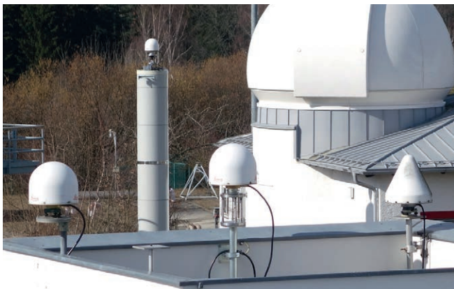
Measuring platform with GNSS antennas
