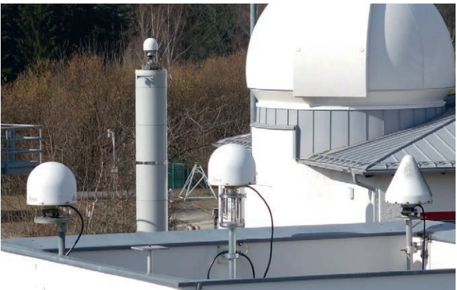
Measuring platform with GNSS antennas
