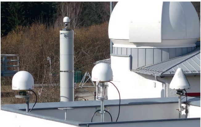
Measuring platform with GNSS antennas
